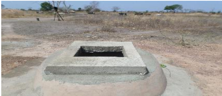
A shallow well created to support access to water in Alok Boma
